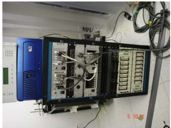
Figure 4. Shows the PT electronics rack with the 8 channel motion controller, a Windows test PC, camera controller, network power switch, four 1U Dell PCs and two RAID disks.
