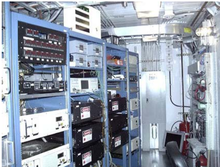
Figure 6: Laser Room Equipment
